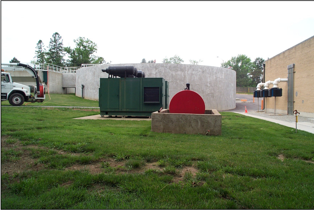
Figure 1: WWTP backup generator diesel fuel secondary containment
