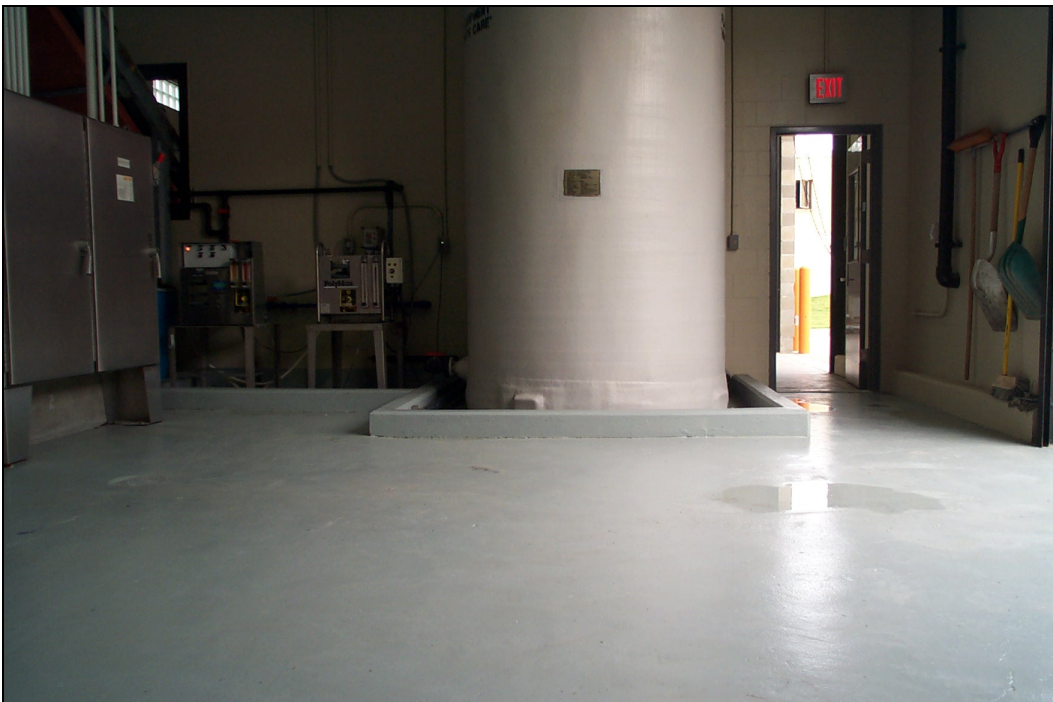
Figure 2: WWTP Class A sludge process polymer storage secondary containment
