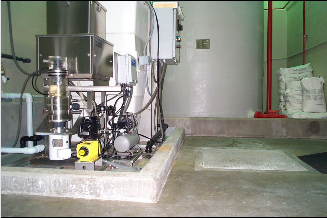
Figure 3: WWTP Actiflow treatment process polymer storage secondary containment
