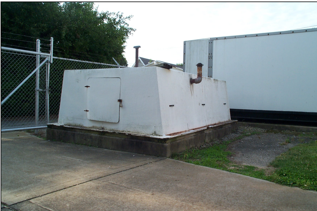
Figure 4: Water Department backup generator diesel fuel secondary containment
